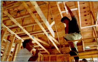
C.S. Monroe Technology Center's building construction program teacher Andrew Campbell gives Timmy Carter, a graduate of Heritage High School, some tips on installing a tray ceiling. Students in the program have been hard at work all year constructing a full-sized home in the Dulles South area along Gunn Spring Road, and have been responsible for almost every aspect of the construction of the house. Once finished, the house will be sold to help fund the next home-building project.
